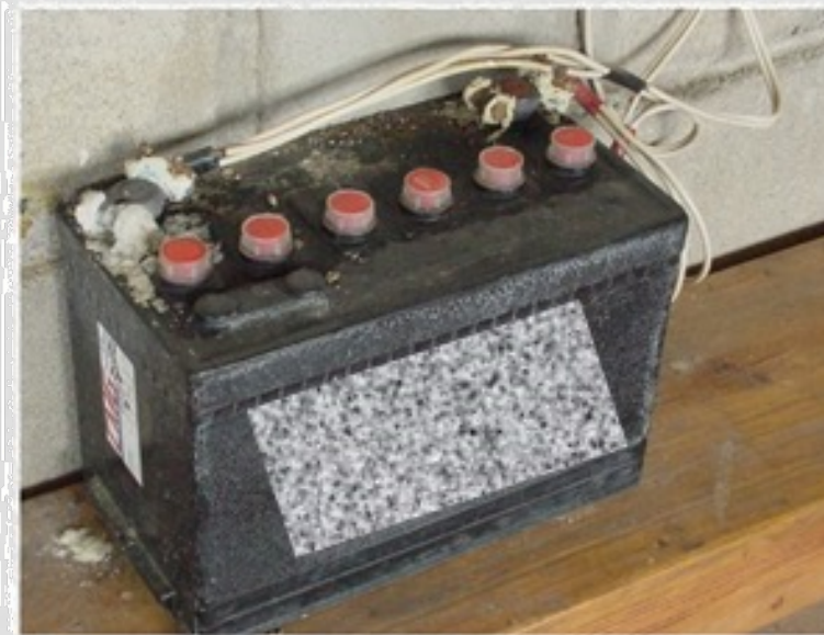
Poorly maintained “self-regulating” system. Note corrosion of terminals!
